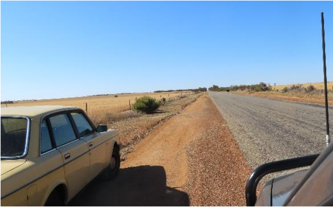
Photograph 2 : A section of the west side of McGregor Road that was recorded from a vehicle rather than walking due to the high level of degradation
